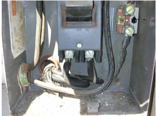
Interior of main disconnect. Old rubber insulated wiring.
